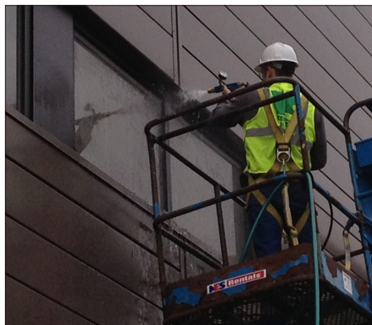
Water Leakage Field Check
